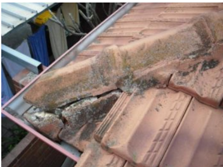
Hip capping deficient
