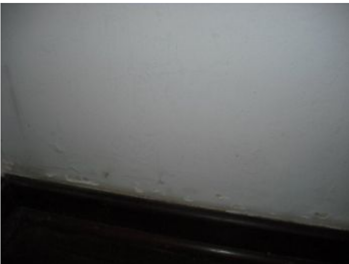
Dampness in walls
