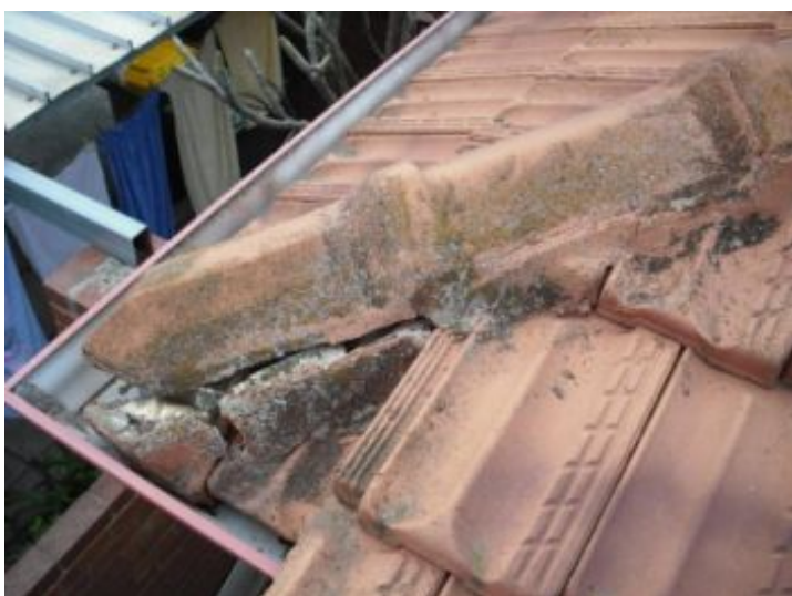
Hip capping deficient
