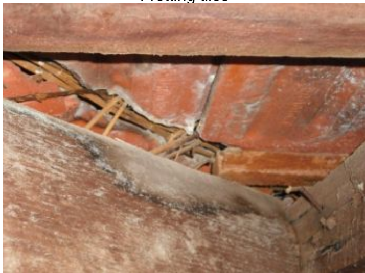
Vine in roof space
