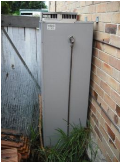
Gas storage hot water system
