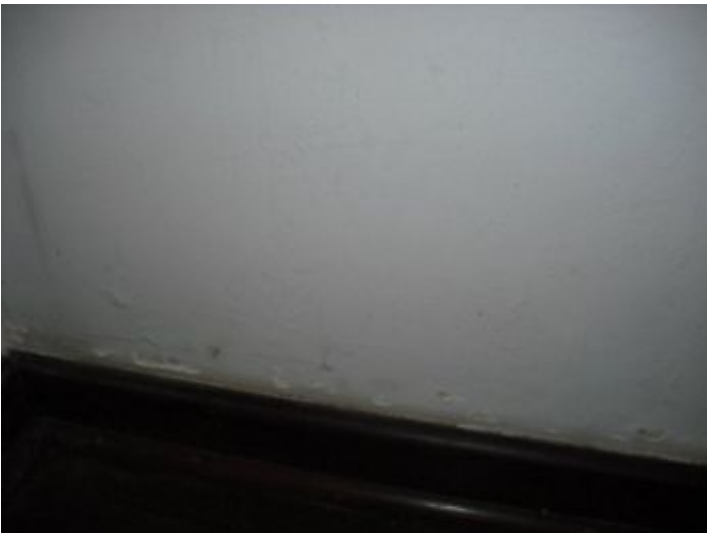
Dampness in walls
