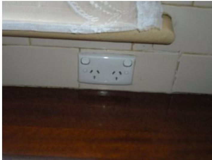
Loose power point
