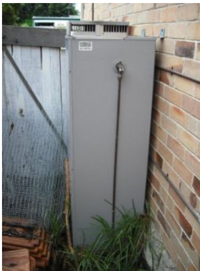
Gas storage hot water system
