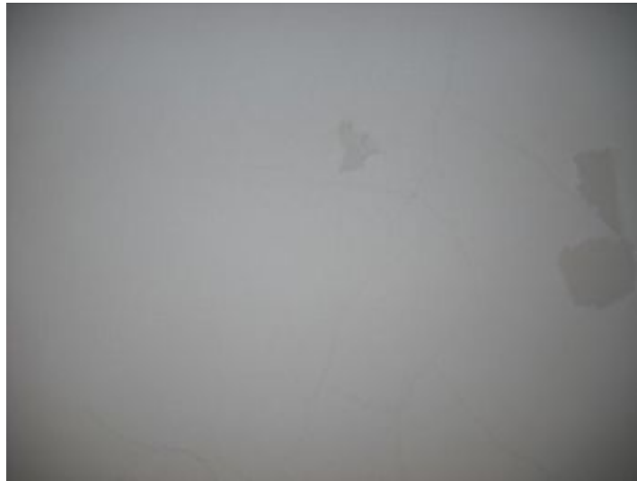
Old water stains
