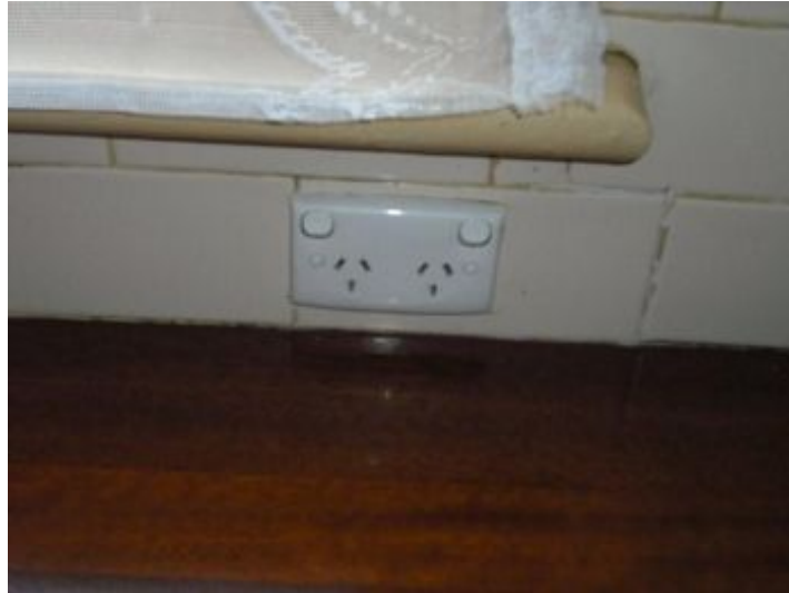
Loose power point
