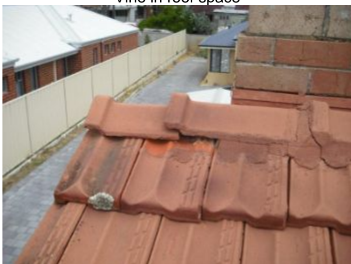
Ridge capping deficient
